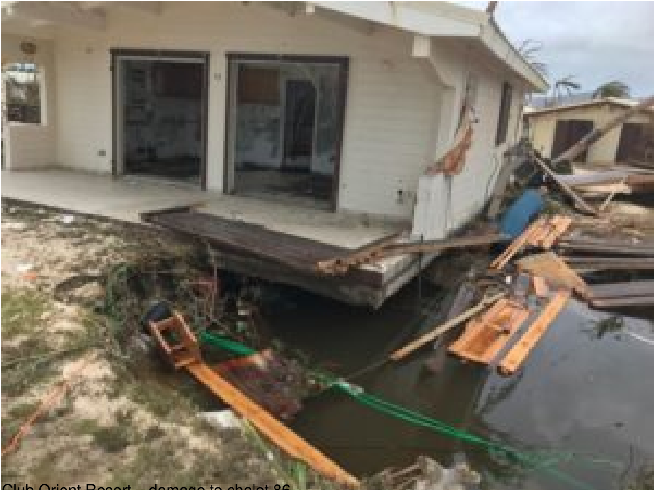
Club Orient Resort – damage to chalet 86
