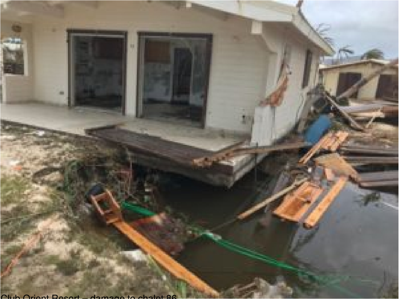
Club Orient Resort – damage to chalet 86
