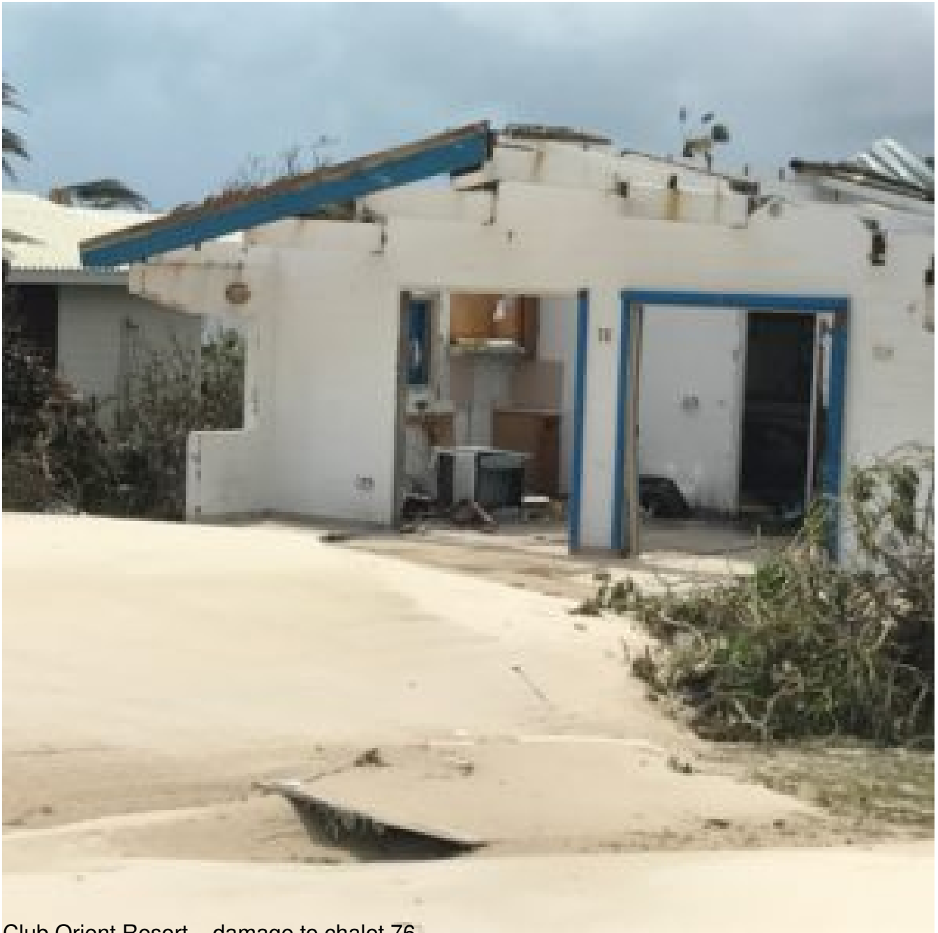
Club Orient Resort – damage to chalet 76
